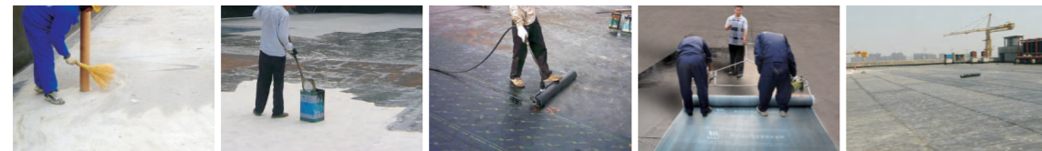
1. Treatment substrate 2. Paint substrate agent 3. Hot melting construction 4. hot material construction 5. Complete spreading and paving
